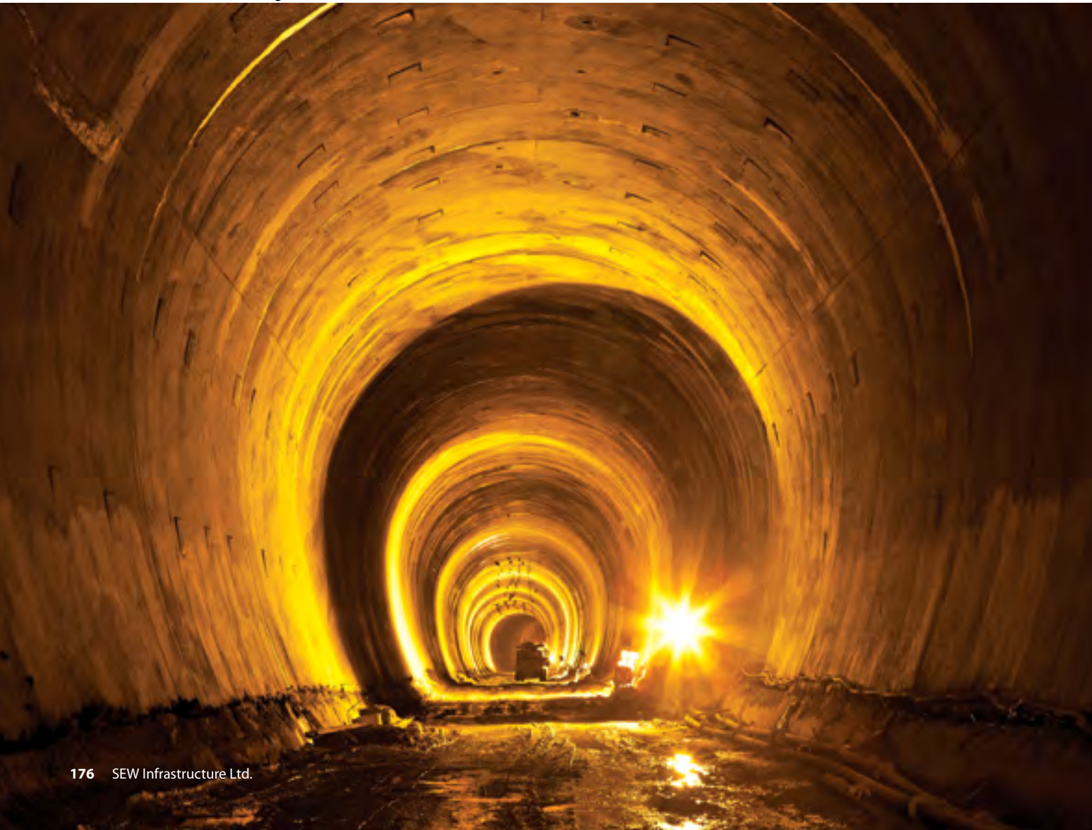
Diversion Tunnel - Teesta Stage III HEP, Sikkim
