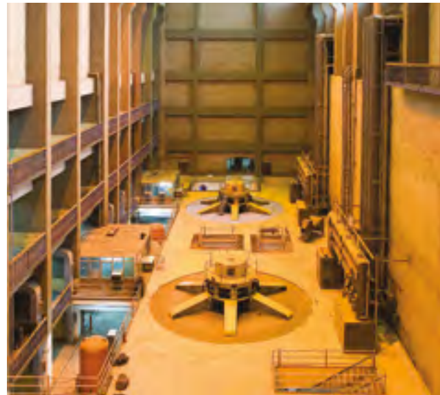
2 x 45 MW Turbine Hall
