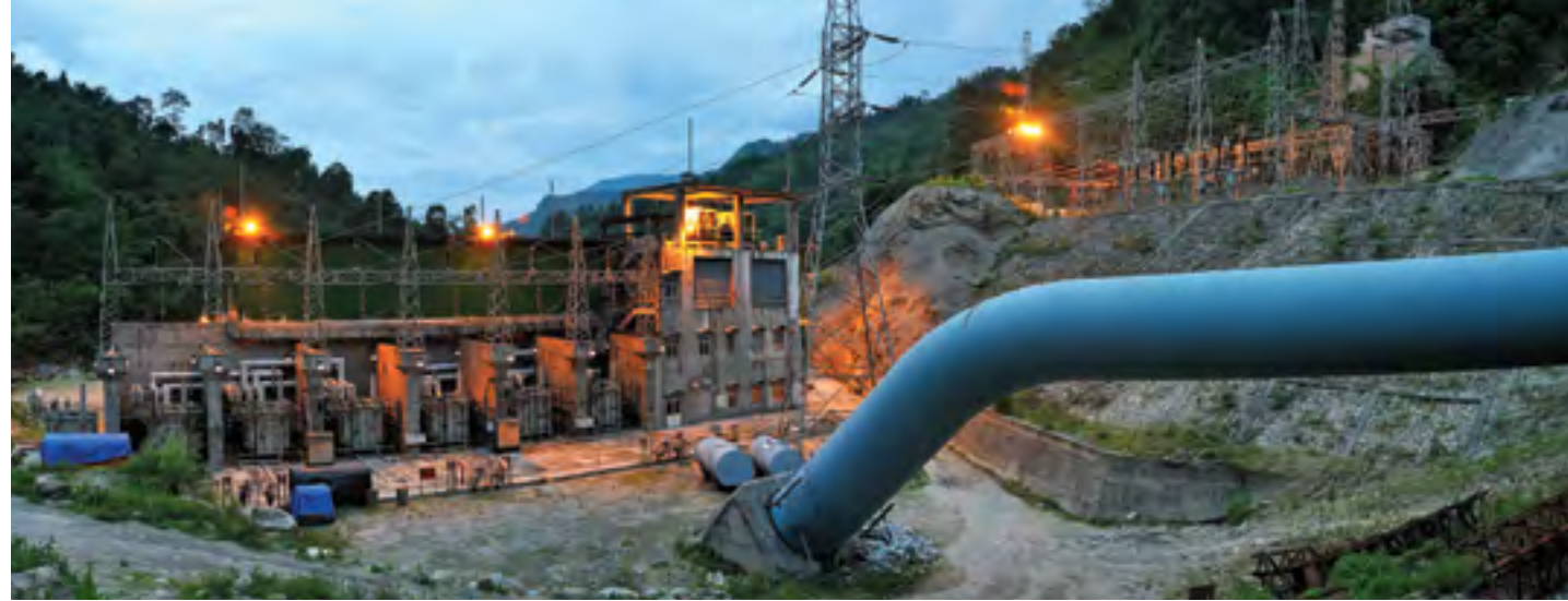
Power House, Penstock and Switchyard
