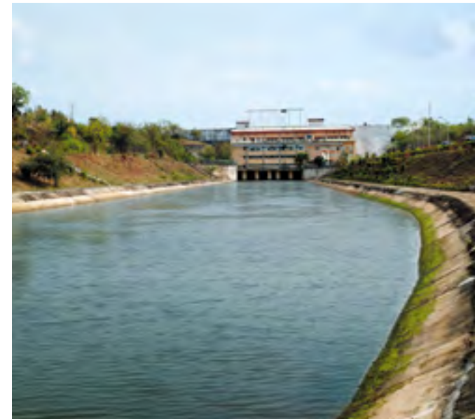
Tawa Hydro Electric Project
