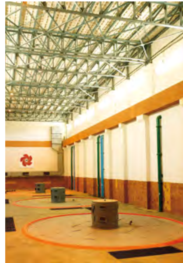
3 x 105 MW Power House Turbine Hall
